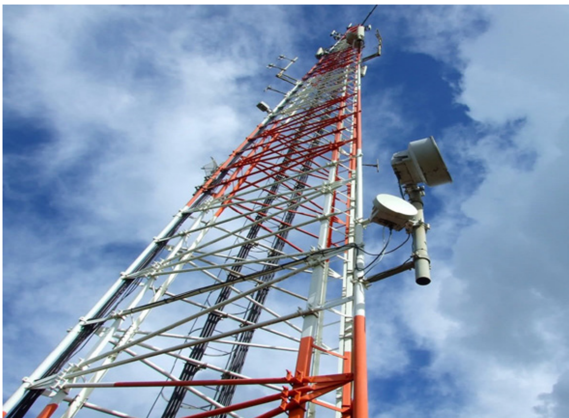
Improved telecommunications infrastructure.
