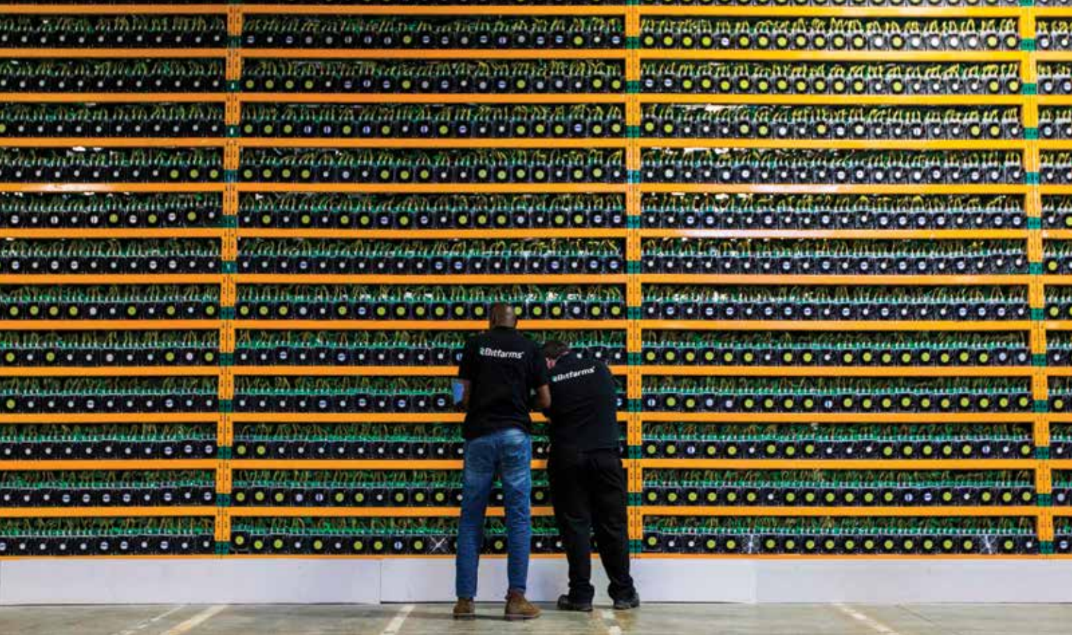
Technicians inspect equipment at a bitcoin mining facility in Quebec, Canada.
