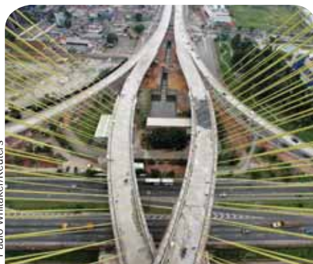
Construction of the Octavio Frias de Oliveira Bridge in São Paulo. Crisis is “stress testing” Latin America.
